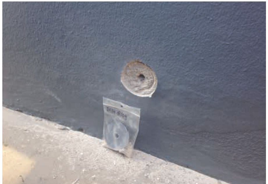
17. In 2018 TNO and Stichting Restauratie Atelier Limburg took samples from specific areas of the exterior and the interior of the Rietveld Schröder House. The photograph shows a sample from the balcony wall on the east elevation (photo author)
