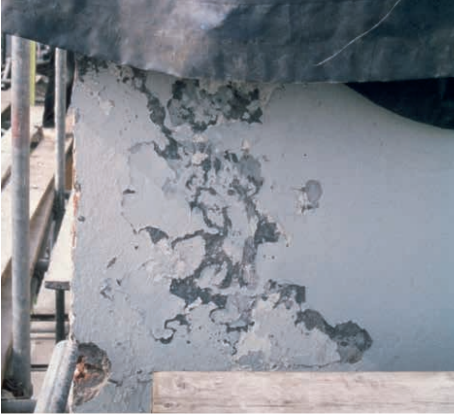
9. In several places, such as here on the chimney, Bertus Mulder discovered various remnants of render and finish coats (Bertus Mulder archive)
