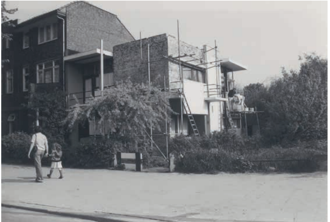
5. In 1979 the Rietveld Schröder House was once again scaffolded after the reappearance of the problems with the plasterwork. Large areas of render were first chipped away, after which a new coat was applied (Bertus Mulder archive)
