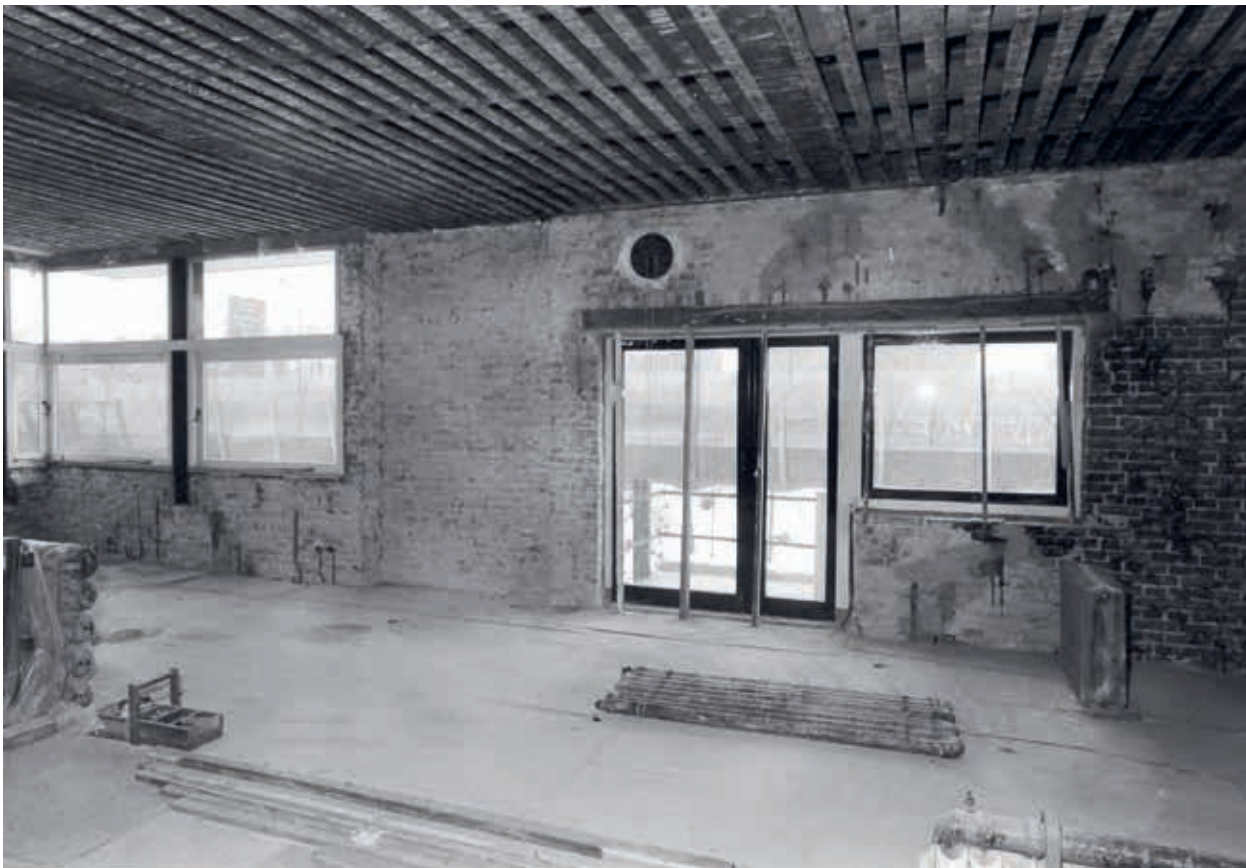
14. During the restoration of the upper floor of the Rietveld Schröder House in 1985-1986, Bertus Mulder completely stripped the walls and ceiling (Bertus Mulder archive)
