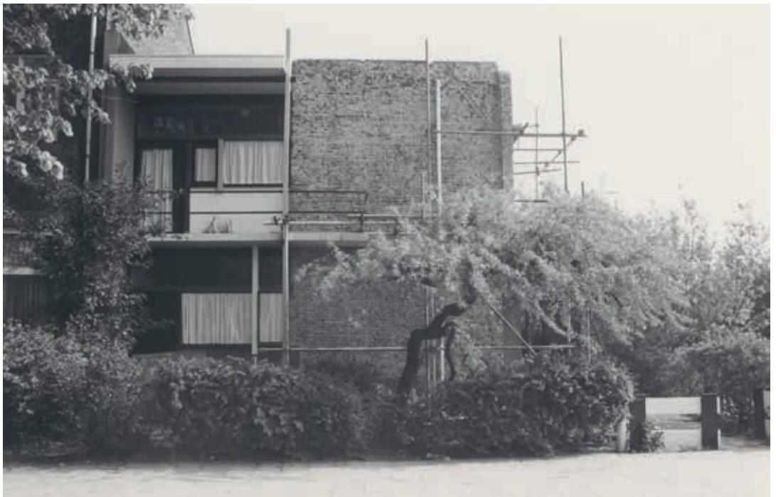
6. The bare brickwork of the wall on Prins Hendriklaan in 1979. On the wall below the window of Rietveld's former studio (bottom left) render is still visible (Bertus Mulder archive)
