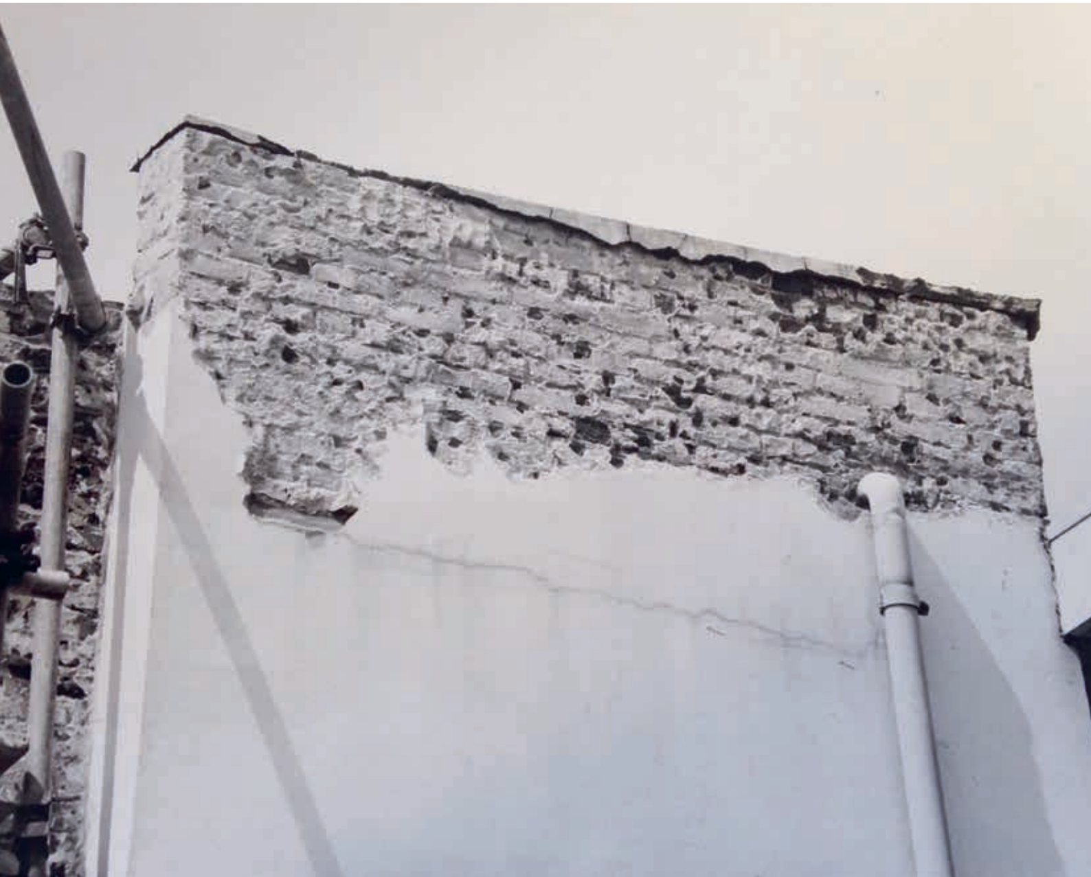
7. Only the render on the upper part of the white wall beside the front door of the Rietveld Schröder House was chipped away in 1979 (Bertus Mulder archive)
