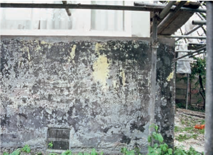
10. Various shades of grey came to light on the window below the kitchen window. Bertus Mulder based the grey for this surface on the dark grey in the top right corner (Bertus Mulder archive)
