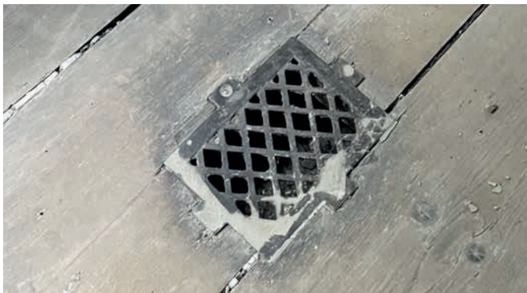
7. Inflow grille for warm air integrated into the floor (photo Matthijs de Kraker, wdjArchitecten)
