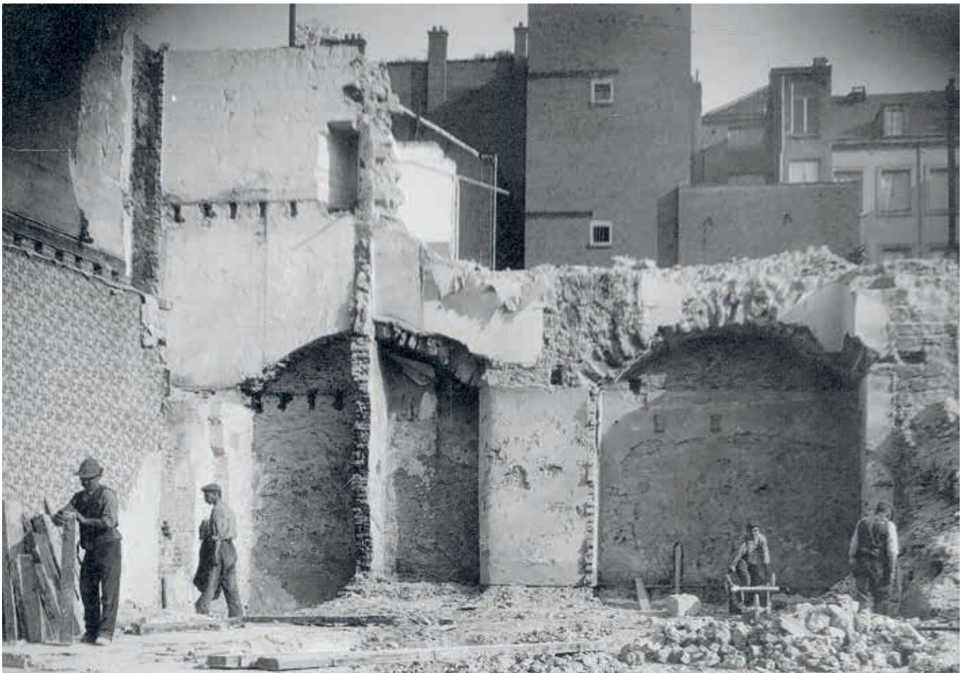
8. The processing and transport of disassembled timber planks and bricks c. 1905 (photo Comité d'Etudes du Vieux Bruxelles, KIK-IRPA, Brussels)
