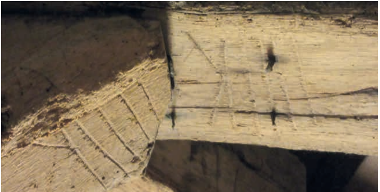
12. Detail of the oak entablature in the northwest tower of the Great Hall. The assembly mark IIIIK has been scribed on the upper side of the corner brace and on the soffit of the beam in the upper horizontal framework (photo H. Hundertmark, 2021)
