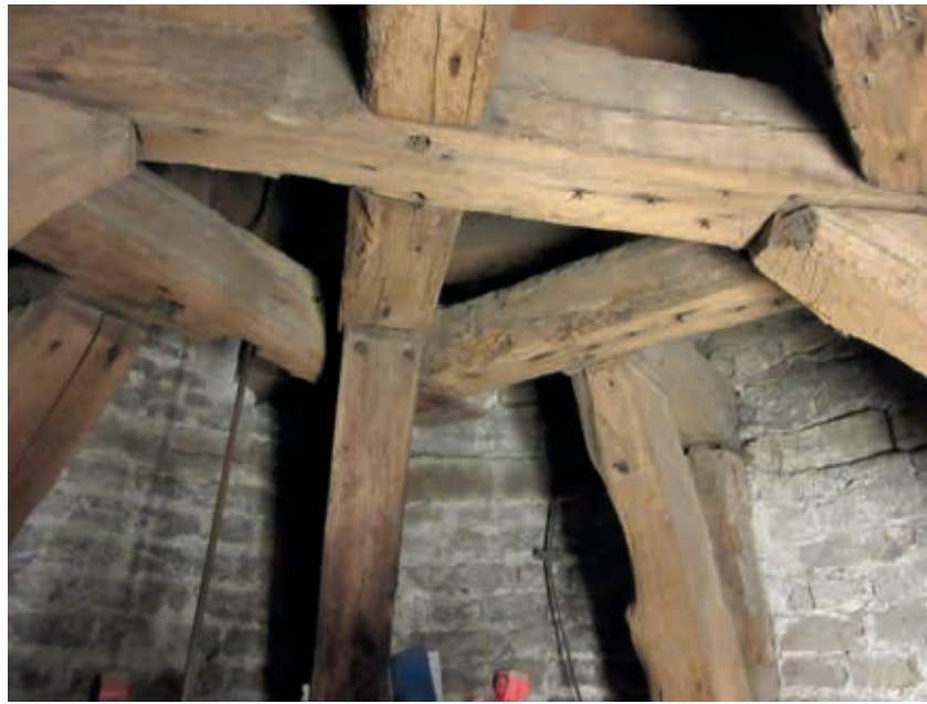
8. Upper horizontal framework of the entablature in the northwest tower of the Great Hall. Scribed assembly marks are visible on the beams. The oak entablature was constructed in 1295 and originally supported a spire (photo H. Hundertmark, 2021)
